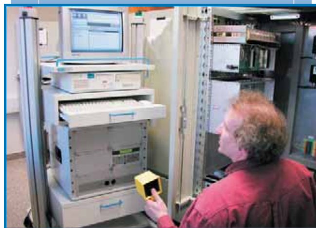
Voltage control of the cabinets
